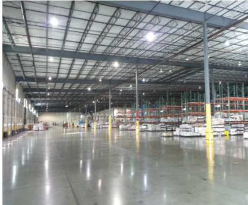
BEFORE - 400w HID consuming 458 watts per fixture
