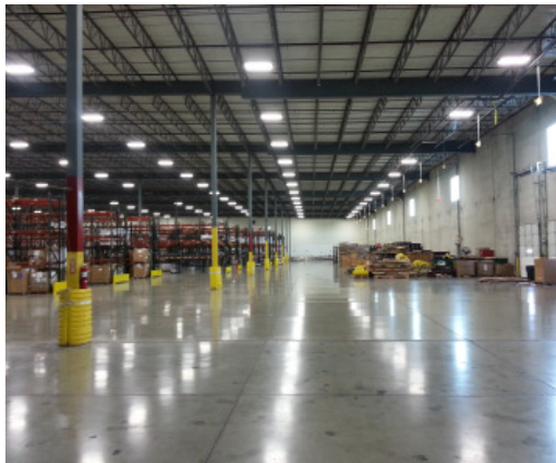
AFTER - 6-Lamp T8 consuming 218 watts per fixture
